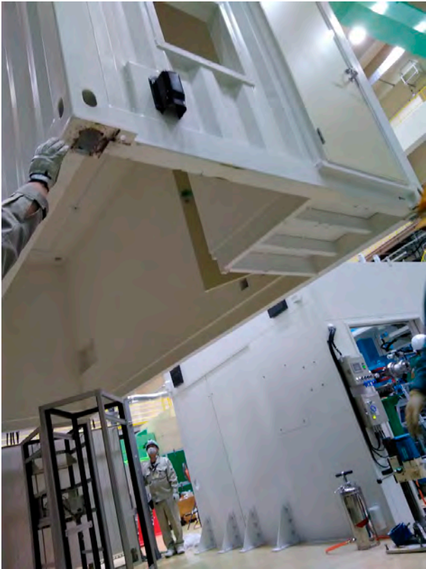
Figure 3. The laser hut hoisted with a crane. Large instruments like a laser table can be installed by moving the hut to another place.
