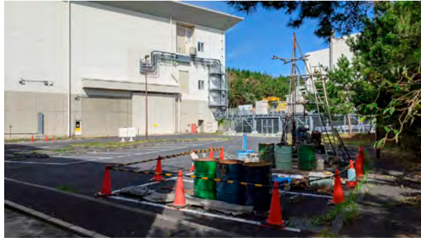
Figure 3. Geotechnical investigation of the construction site of the extension building for the H2 area.
