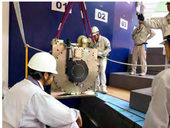
Figure 1. The new T0 chopper being installed on 4SEASONS.
