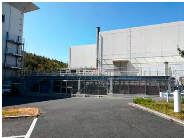
Figure 1. Electric power substation constructed on the east side of the MLF building (left). The white wall in the back is that of the NU2 building (Photo taken in May 2019).
