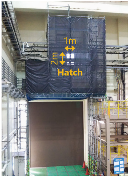
Figure 3. Aperture for the electric transmission lines. It is located above the carry-in entrance of the east #1 experimental hall of the MLF.
