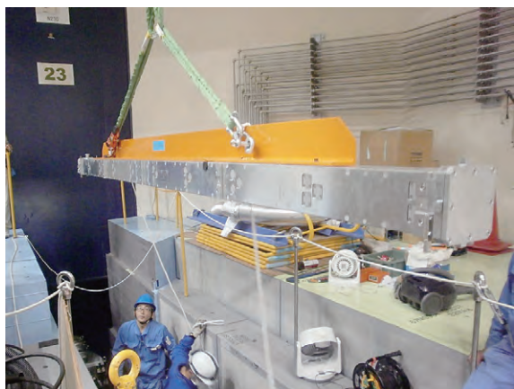
Figure 2. Installing operation of the 4 m super mirror guide tube in the beam line.
