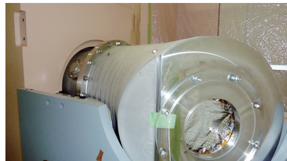
Figure 4. The damaged thermal insulation window was fixed by removing all shields in the vicinity of the superconducting curved solenoid.
