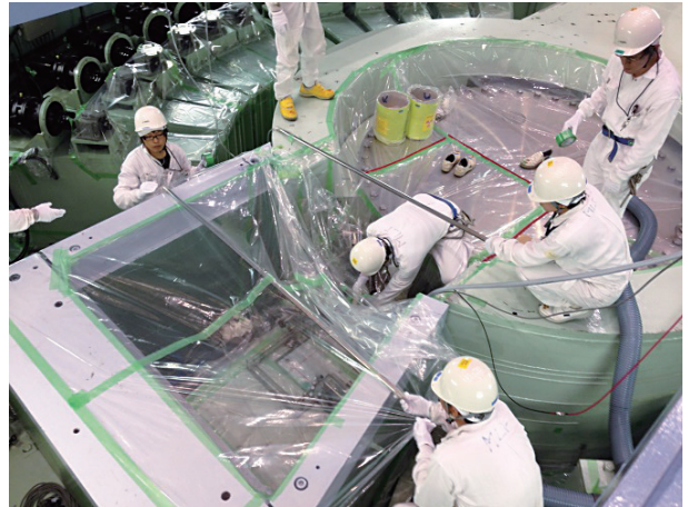
Preparation of local room, called green house, with local ventilation system to prevent from contamination during replacement of the proton beam window.
