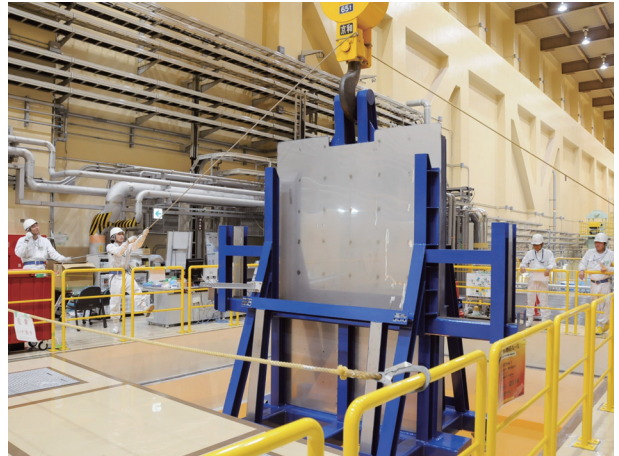
Installation of additional shielding wall to reduce external exposure of worker in a hot cell.
