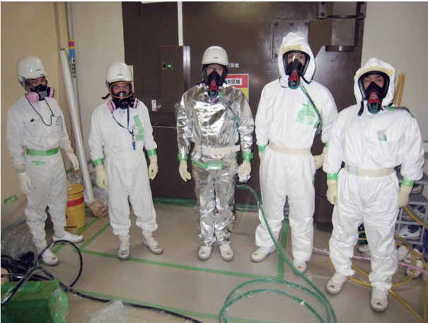
Preparation for mercury discharge. Center person cut and welded helium gas pipe with mercury.
