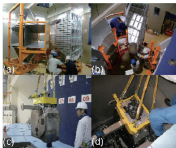
Figure 1. The construction of the SPICA diffractometer (a), (b) and the installation of the T0 chopper (c), (d).
