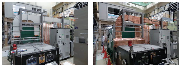
Figure 4. Cable rack for the power cables shielded with copper sheets.
