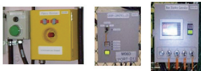
Left : Search Button Right : Panic Button Door Controller Blocker Controller
