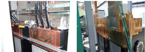
Figure 2. The feed-through terminals enclosed with copper sheets.
