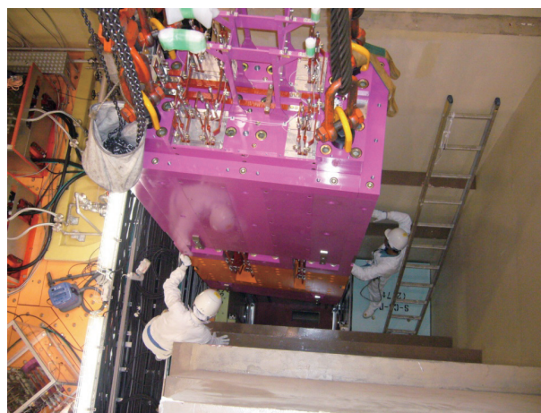
Figure 2. Installation of the SQ4-5-6 triplet magnet.
