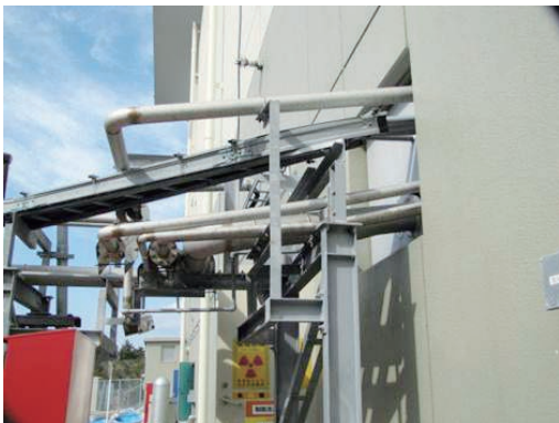
Figure 1. Damaged helium ducts for the on-line refrigerator at the boundary of the MLF building.
