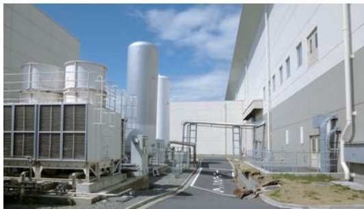
(a) After the earthquake (Mar.)
