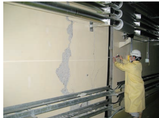
Figure 2. Collapsed wall by the Great East Japan Earthquake at the expansion joint in the tunnel.
