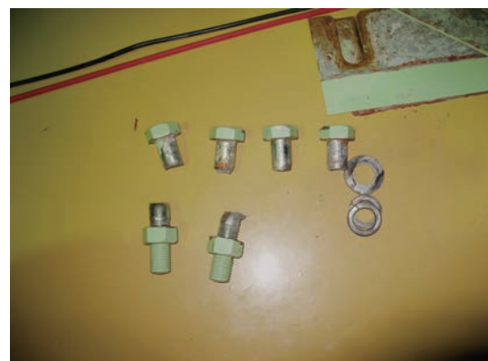
Figure 3. Broken bolts for the rail of the suspension crane due to the vibration.
