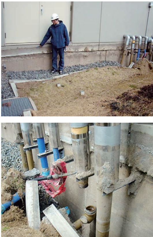
Figure 1. Ground surrounding the MLF building subsided ~1 m (top) and the pipes of the water supply and water drain were torn off.
