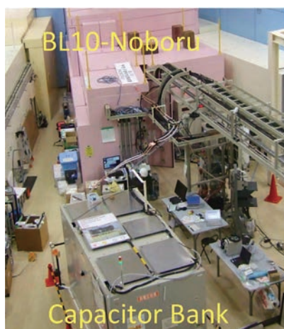
Figure 1. 250 kJ Capacitor bank set at MLF.
