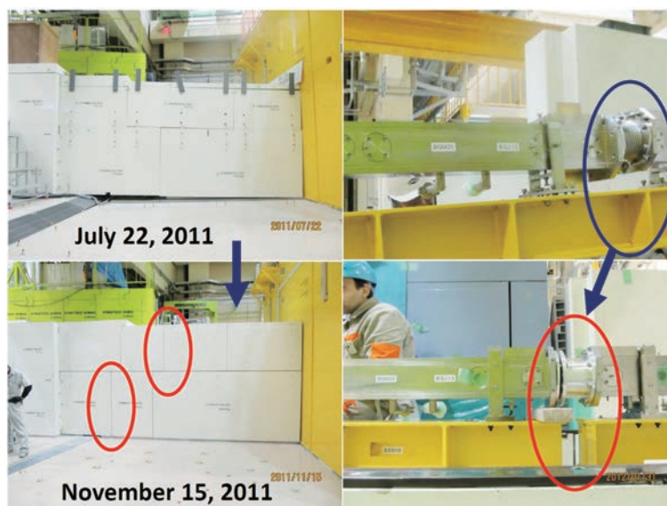
Figure 10. The lessons learned from the earthquake disaster. The separated beamline shields (left) and the separated neutron guides and the supports (right) around the boundary region between MLF main building and the extension building.
