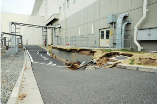
Figure 1. Ground subsidence around the MLF building ©KEK
