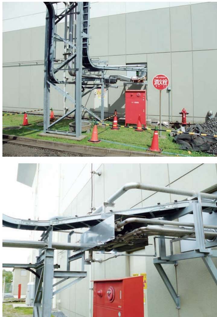
Figure 1. Photograph of the broken He piping for the refrigerator, located just outside of MLF building before (above) and after the repair (below)
