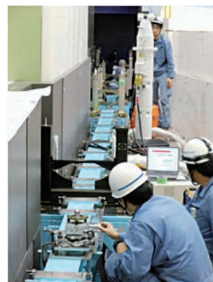
Figure 2. The alignment works of super mirror guide in BL02 beam line by laser tracker. (October 22, 2011)
