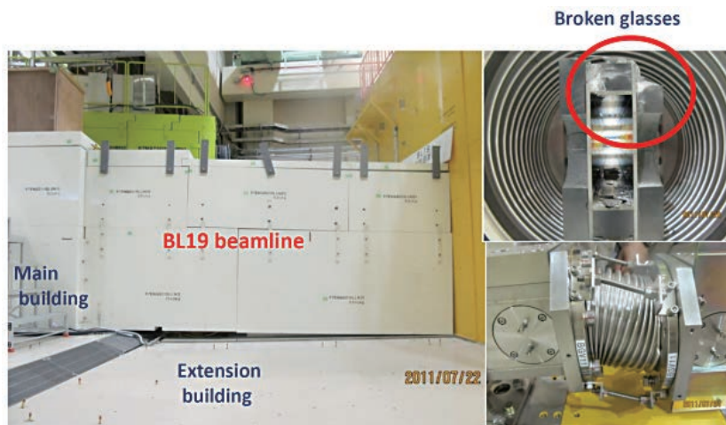
Figure 9. Overview of the inclined shields (left) and the broken glass of the neutron guide mirror (upper-right) and the tilted bellows of the neutron beamline (lower-right).
