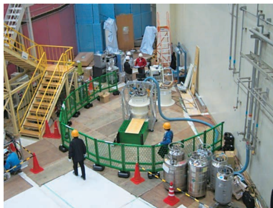
Figure 1. Test operation of the 7 T vertical-field superconducting magnet, performed at the MLF experimental hall 2 in March 2012.
