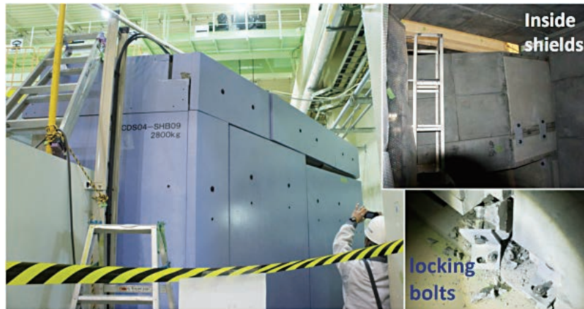
Figure 7. Outside view of neutron shields around the SENJU diffractometer (left) and the inside (right). The shields were partially damaged and tilted. The locking bolts of the shields were broken.
