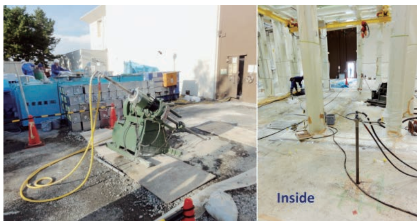
Figure 4. Grouting (injection of low-viscosity grout) for ground improvement at outside and inside the extension building.
