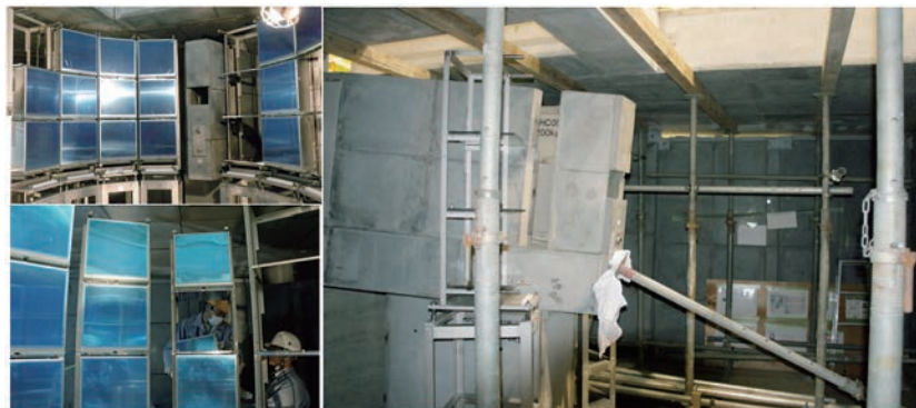
Figure 8. Two-dimensional detectors (left) and the reinforced inclined-shields (right) in the shield room of SENJU diffractometer.
