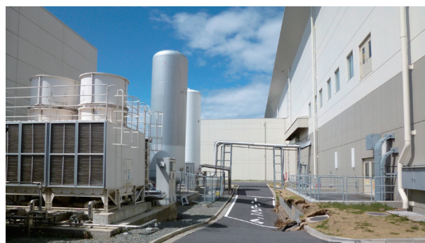
Figure 7. Condition of the tanks and the pipes of the cryogenic system outside of the MLF building.
