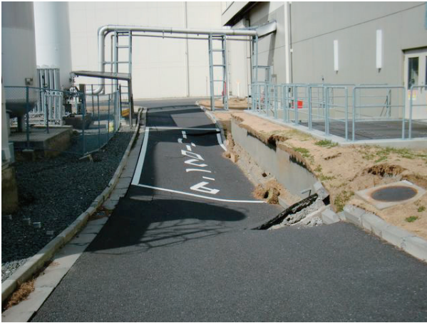
Figure 4. Subsidence at the southeast part of the MLF building.
