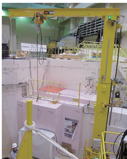
Figure 4. A jib crane newly installed at AMATERAS
