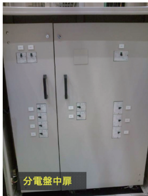
Figure 2. Electric power supply newly set at the SE handling area.
