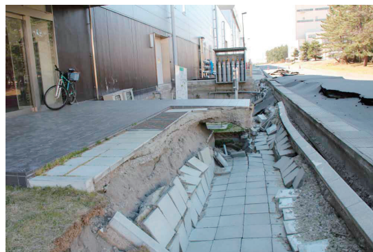
Figure 2. Subsidence at the Linac entrance.
