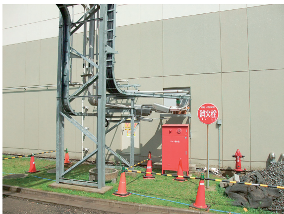
Figure 1. The broken He piping for the refrigerator, which is located just outside of the MLF building.
