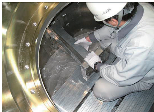
Figure 6. Installation of a Cd beam duct and a beam narrower in the scattering chamber.
