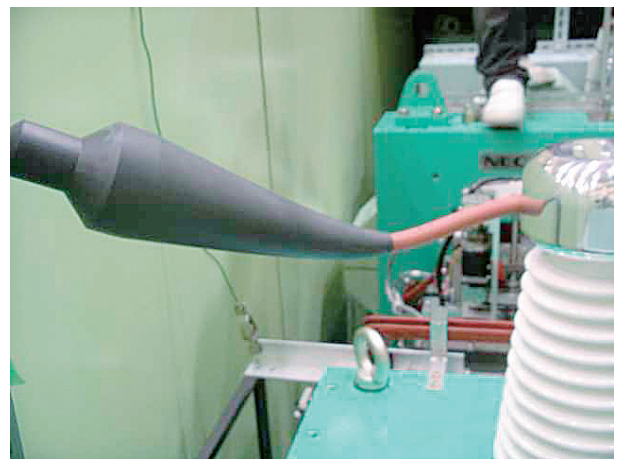
Figure 1. The cable terminal of DC-separator.
