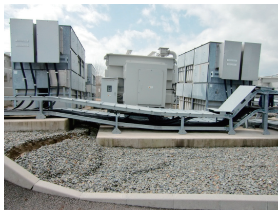
Figure 3. Subsidence at the 3-GeV power supply yard.
