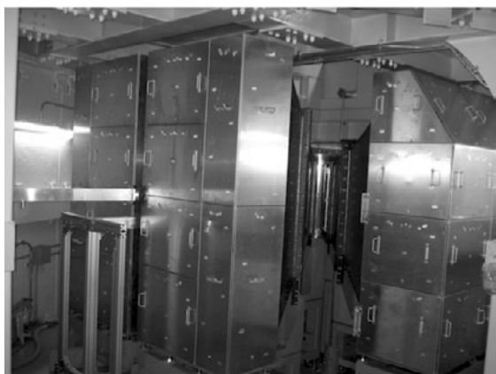
Fig. 5 A new SuperHRPD chamber was installed in summer of 2009.
