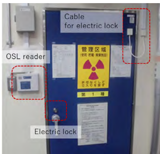
Figure 1. Electric lock and OSL reader authorizing the entry to the controlled area at the BL22 building.
