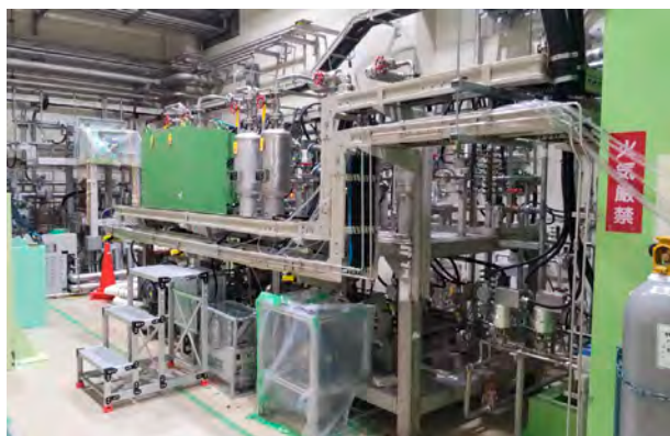
Figure 1. Photo of the off-gas processing system.
