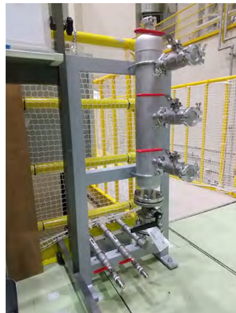
Figure 3. Utility rack of cooling water and helium gas recovering lines added on the shielding house.
