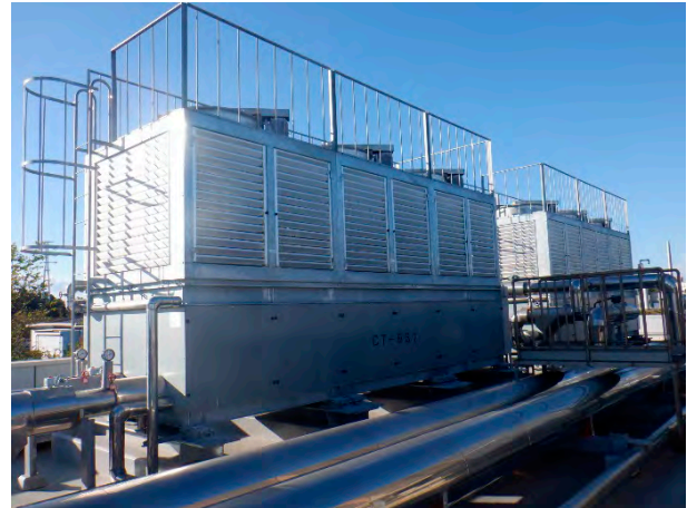
Figure 3. Chilled towers of the 3NBT water cooling system.
